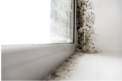
Damp and Mould
